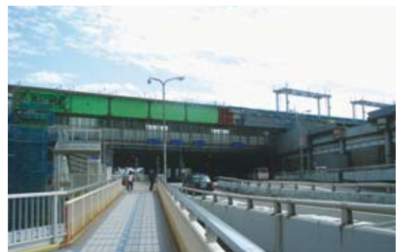
Construction Project of an Elevated Bridge in the Construction Section at Shin Osaka Station
